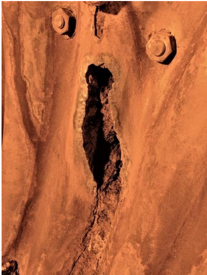
Figure 3: Example of corrosion damage noted internally in galvanised steel culvert.
